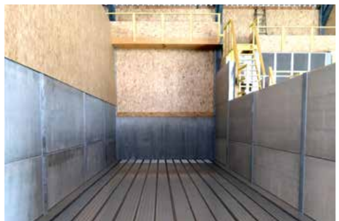
Hay drying system with combined drying floor for drying various bulk materials.
